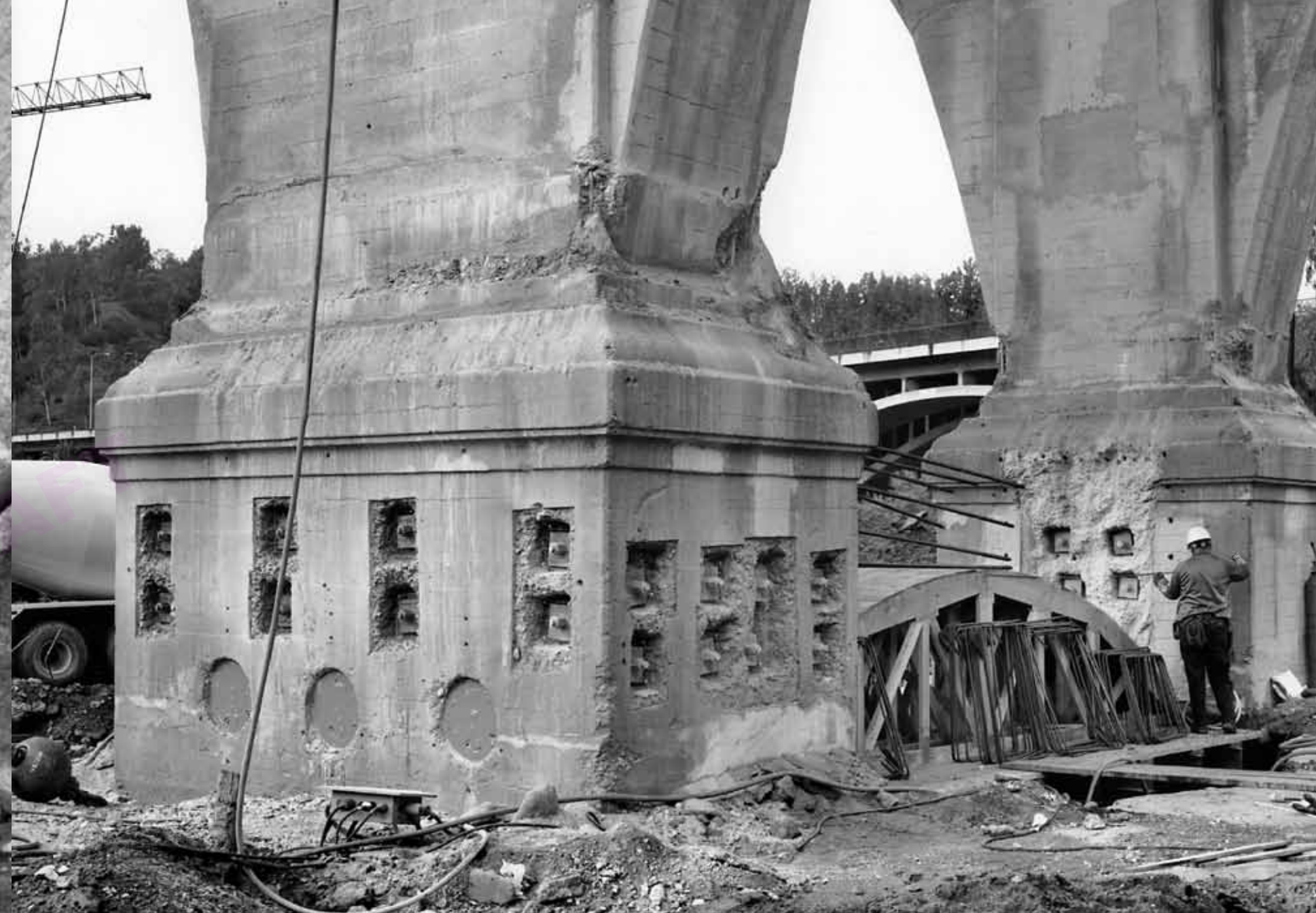
STRENGTHENING OF THE MAIN BRIDGE PIER BASES WITH HIGH STRENGTH STEEL RODS AND RECONSTRUCTION THE CONCRETE STRUT.
