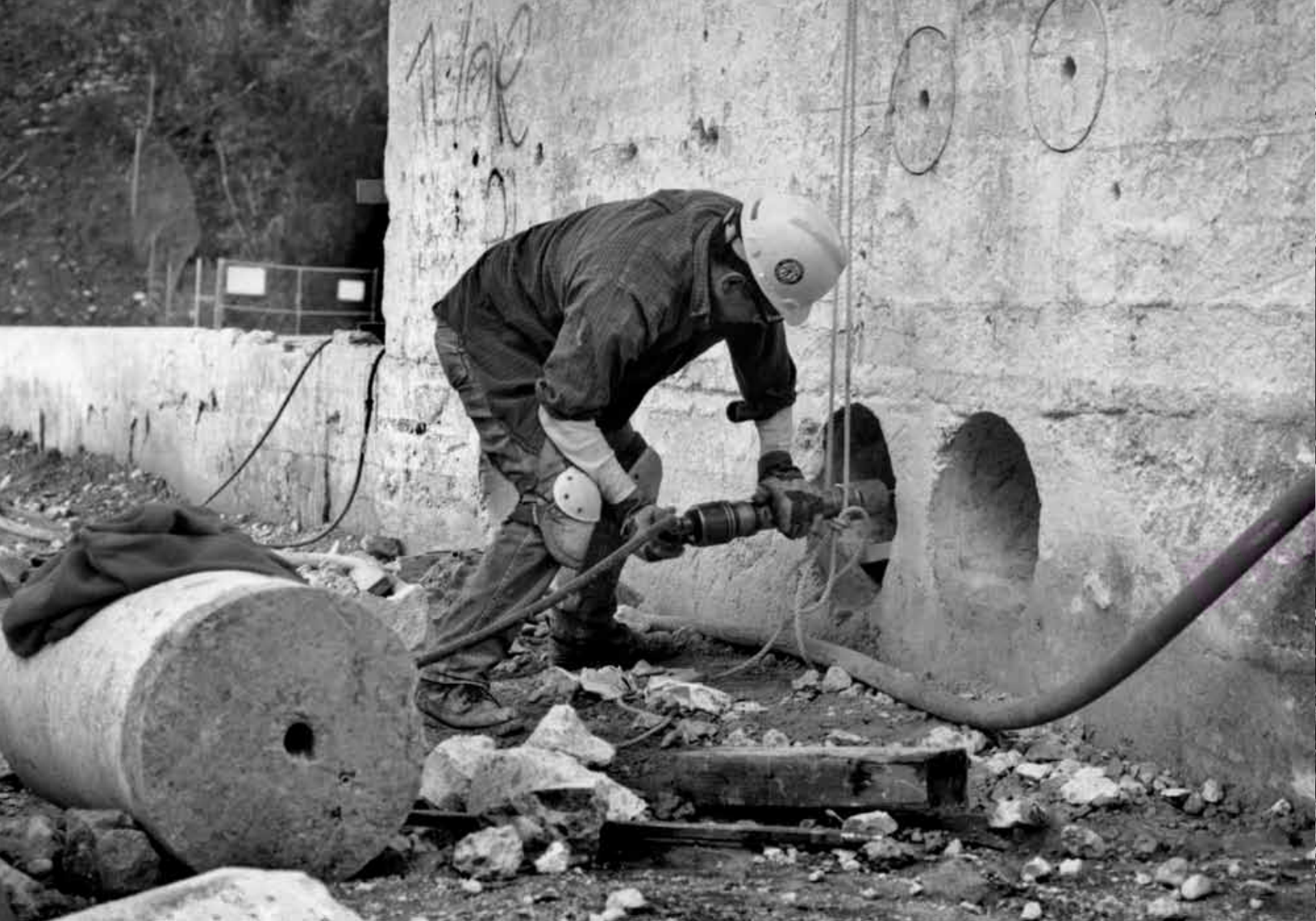
CUTTING ACCESS THROUGH THE COLCROFT PIER BASES TO INTERCEPT THE VERTICAL HIGH STRENGTH WIRDS.
