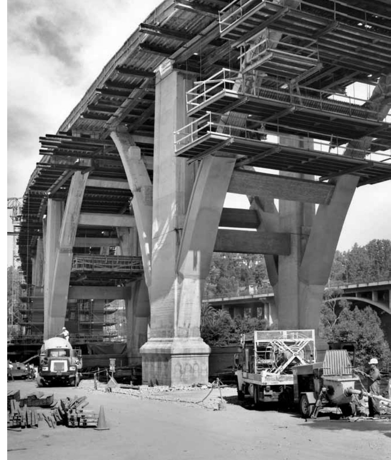
SCAFFOLDING AROUND UPPER PORTIONS OF ARCHES AND STRUTS PROVIDE ACCESS FOR THEIR RESTORATION.
